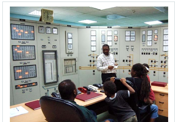
Inside hydropower plant facilities in Tanzania.
