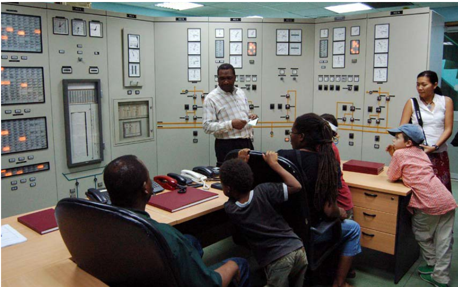
Figure 3. Inside hydropower plant facilities in Tanzania. Photo credit: Paul Shaffner via Flickr [CC BY 2.0 ( https://flic.kr/p/3bZzV8 )]
