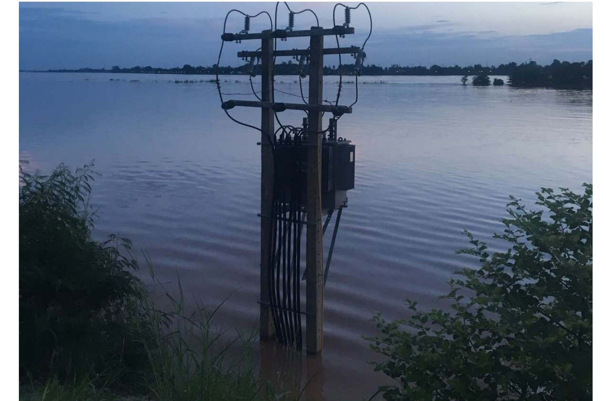
In 2018, flooding in the Mekong Delta caused power outages in the Lao PDR when equipment sited within the flood zone was inundated with rising water.
